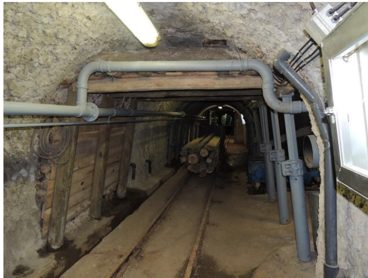
Figure 2: View of the lower drift of 'Marcelo Jorissen Mine' located in the courtyard of the School
